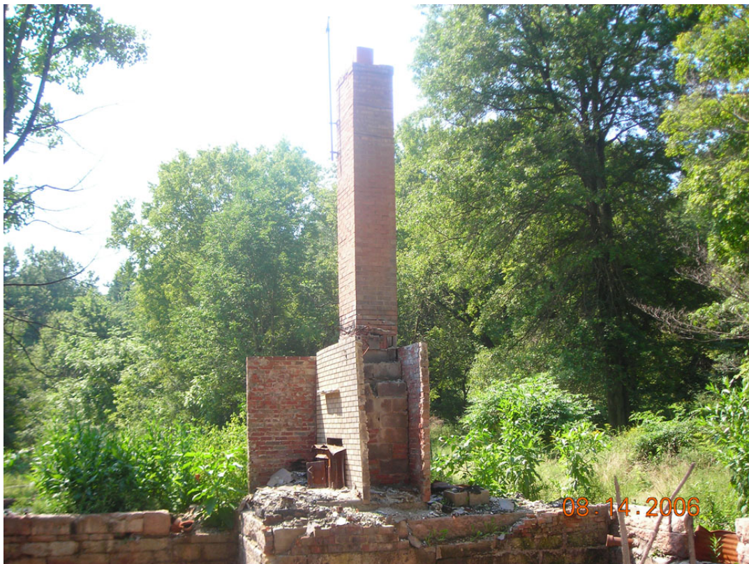
Fig. 123. This is the remains of Biros's home which had been boarded up and sustained fire damage. Eventually the entire home collapsed.
